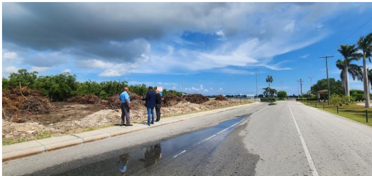
PHOTO SUBMITTED: CIAA CEO Albert Anderson, Minister for Tourism and Ports Kenneth Bryan, and CIAA Board Chairman Johann Moxam visit the site of the new parking facility
